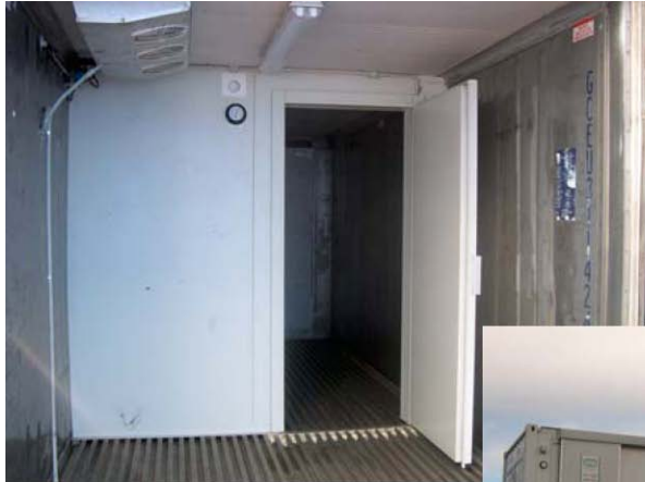
Two zone- freezer and cool room
